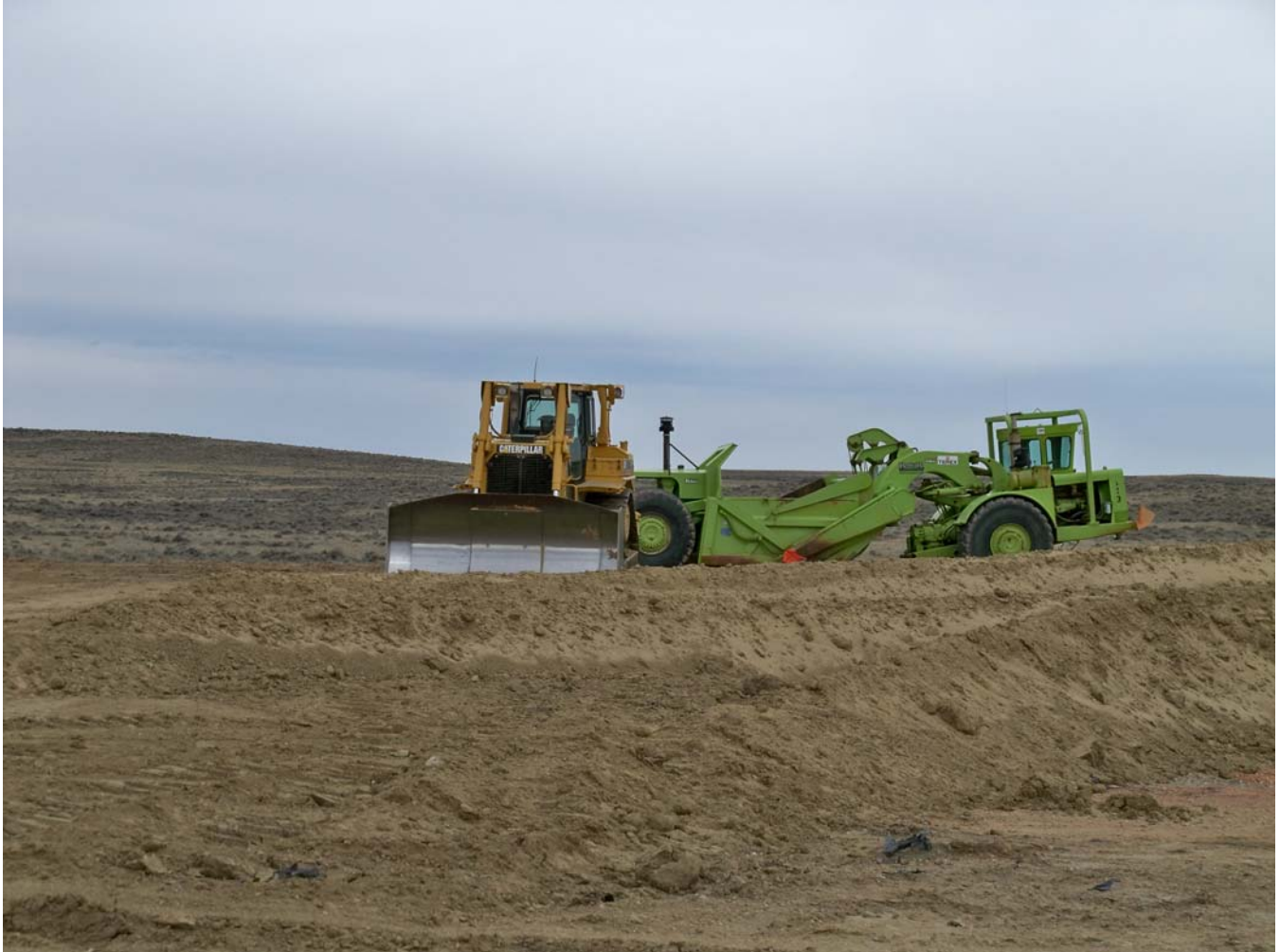
Photograph #2: Evidence of Reclamation
