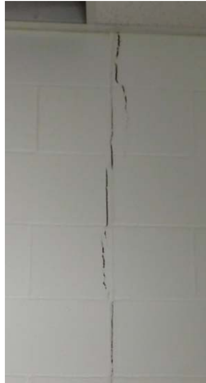
Figure 26B. Vertical crack in north wall of Gymnasium, Room F125, as viewed from Corridor F127.
