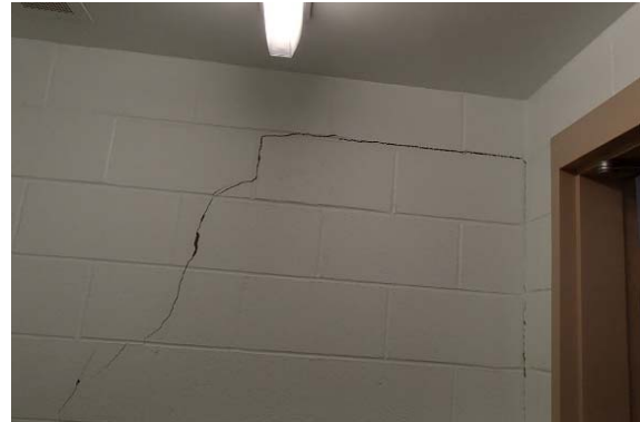
Figure 12B. Cracking in north bearing wall near joint with non-bearing wall in Room B171. WJE Photo P6150269, date 6/15/17
