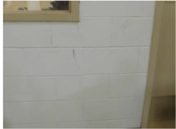
Figure 28B. Masonry cracking in east wall of Room F117. WJE Photo DSCN1267, date 6/15/17
