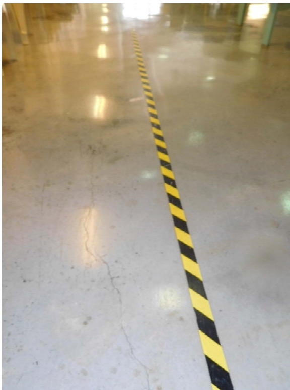
Figure 7. Slab crack in cell Dayroom parallel to front wall of cells
