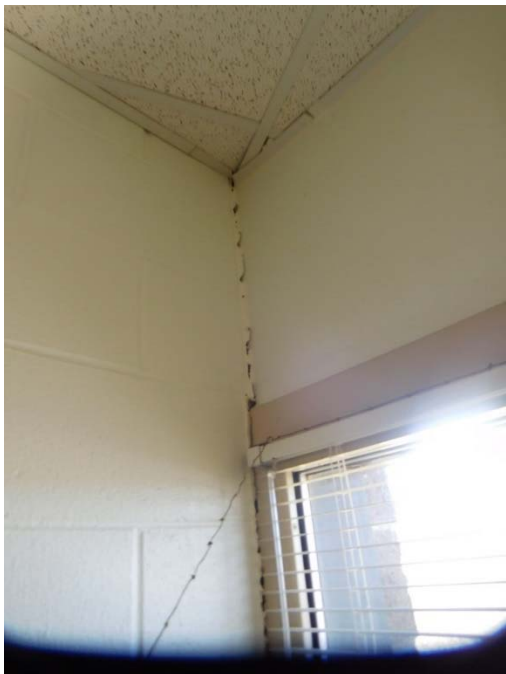
Figure 19. Vertical crack at intersection of non-bearing partition and bearing wall in Room D173
