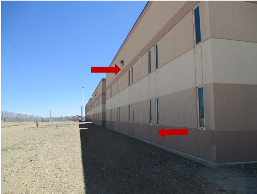
Figure 30. Water staining below windows and at light fixture.
