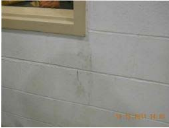
Figure 28A. Masonry cracking in east wall of Room F117. WSP Wall Movement History Rpt. March 31, 2015, page 3 of 141, photo date 12/12/11
