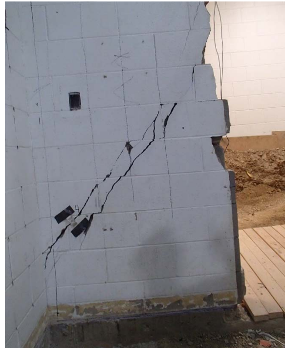
Figure 23B. Cracking in east wall of Gymnasium near NE corner, Room F125. (Note Crack Gauge No. 4 at lower left.)
