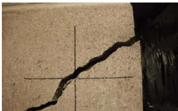
Figure 39A. Fractured masonry pilaster in Mechanical Room 204 in K Unit. WSP Wall Movement History Rpt. March 31, 2015, page 81 of 141, photo date July 2013
