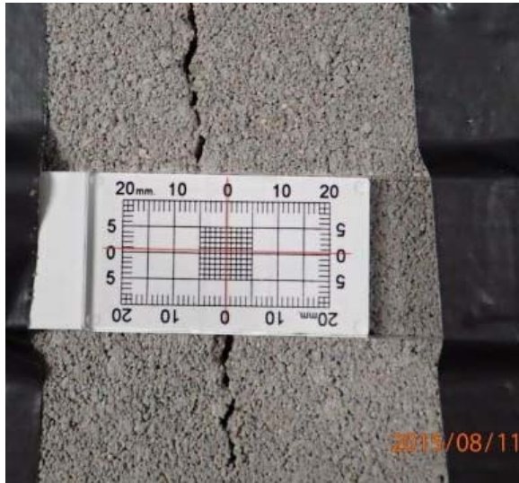
Figure 2A. Crack Gauge 1 - Area F along east wall of Electrical Room F116. M/M WSP Crack Monitor Comparison, page 1 of 4, photo date 8/11/15
