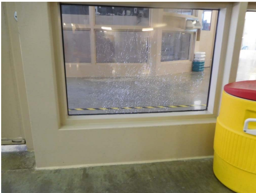
Figure 15. Broken glass window in Pod B rotunda
