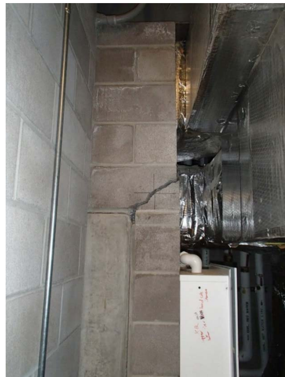
Figure 39B. Fractured masonry pilaster in Mechanical Room 204 in K Unit.
