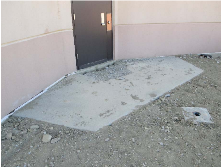
Figure 36. Exterior slab altered to allow egress door to operate.
