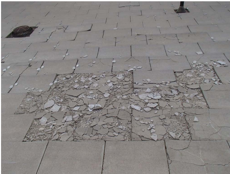
Figure 37. Distressed roofing pavers at South Facility
