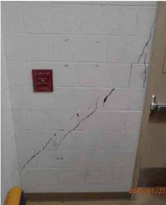
Figure 23A. Cracking in east wall of Gymnasium near NE corner, Room F125.
