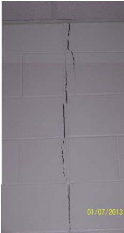
Figure 26A. Vertical crack in north wall of Gymnasium, Room F125, as viewed from Corridor F127. WSP Wall Movement History Rpt. page 67 of 141, photo date 1/7/2013
