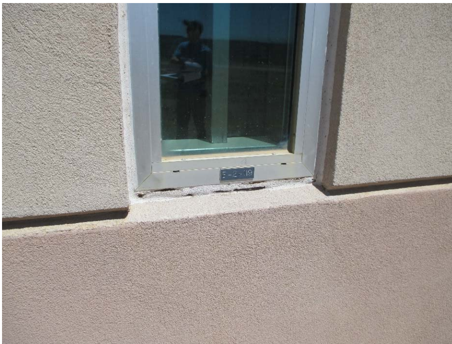
Figure 33. Failed joint sealant at window.
