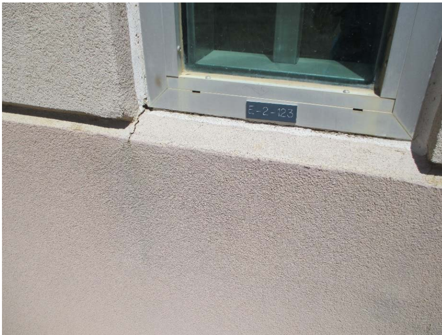
Figure 31. Crack at lower corner of window.
