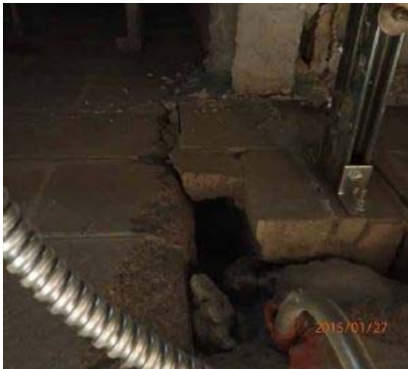
Figure 29A. Distressed masonry beneath steel beam bearing near new column in Corridor F127. M/M Rpt. page 33 of 284, photo date 1/27/15
