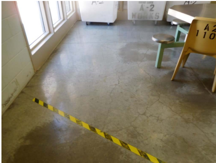
Figure 8. Interior floor slab cracking in Pod A1 adjacent to courtyard
