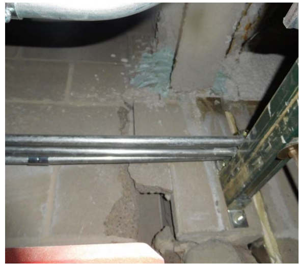
Figure 29B. Distressed masonry beneath steel beam bearing near new column in Corridor F127. WJE Photo DSCN1302, date 6/15/17
