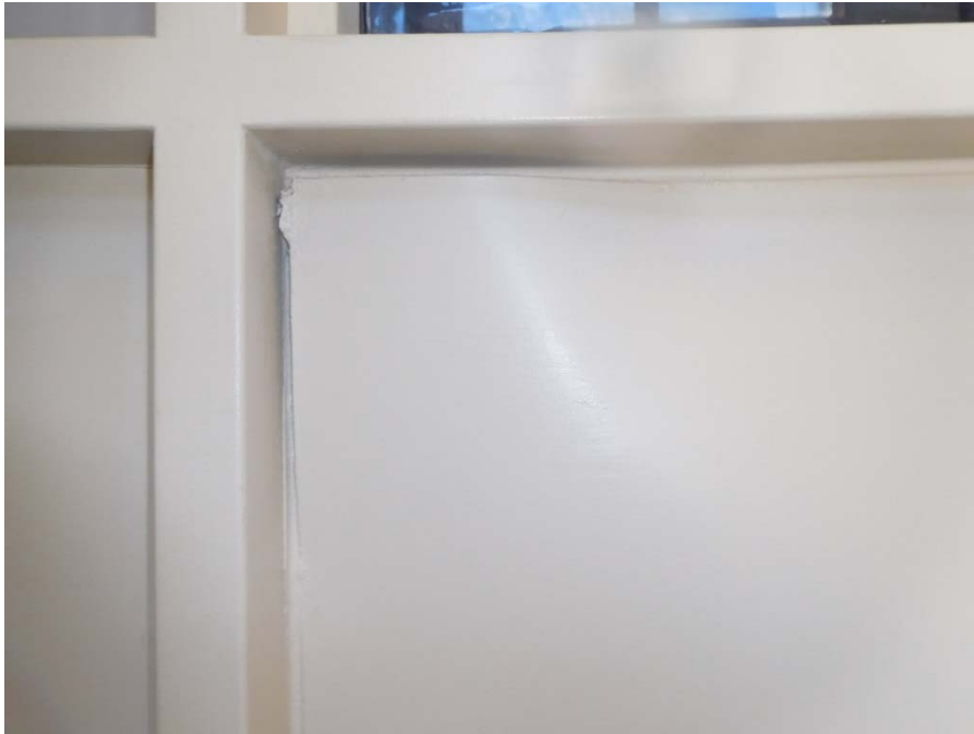
Figure 14. Broken weld and buckled steel plate at Pod B rotunda
