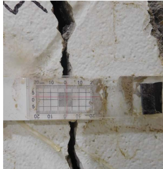
Figure 5B. Crack gauge 4 - Area F near NE corner of Gymnasium, Room F125.
