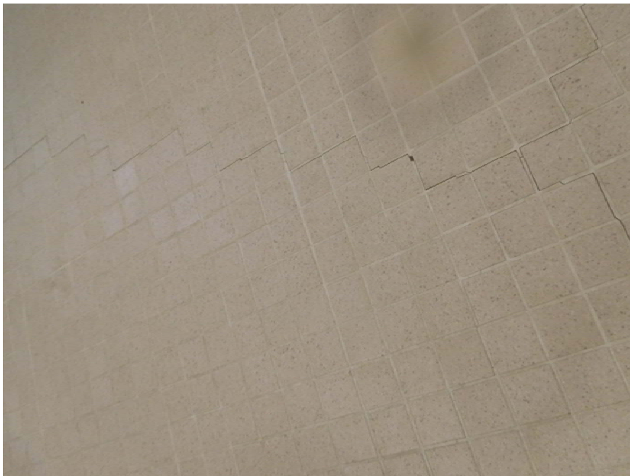
Figure 21. Floor tile cracking in Waiting Area D108
