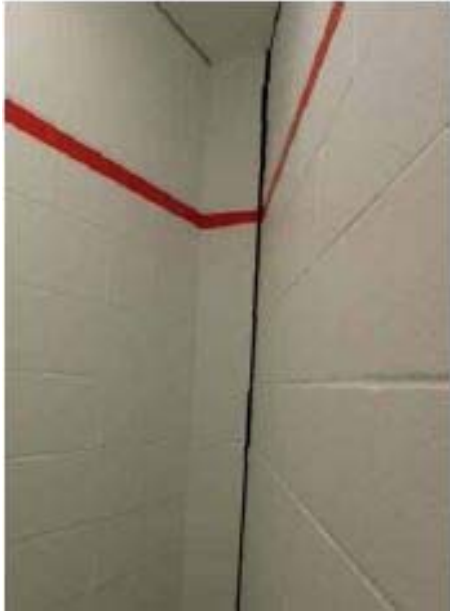
Figure 10A. Separation in masonry at joint between non-bearing (left) and bearing wall (right) in Storage Room A180. M/M Rpt. page 37 of 284, photo date 1/27/15
