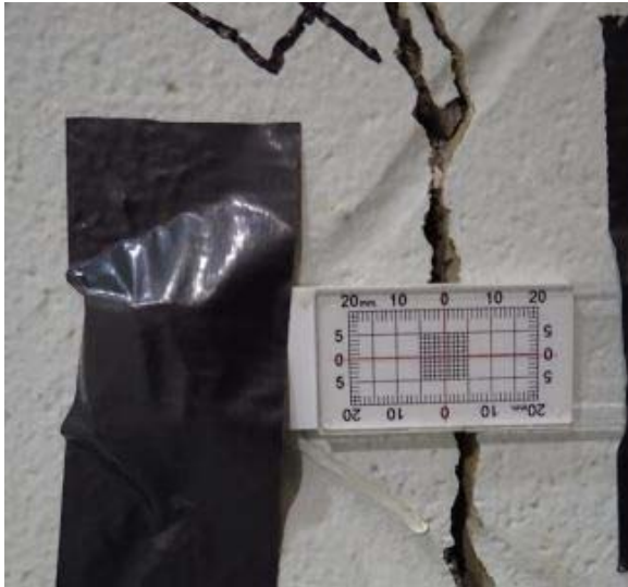
Figure 5A. Crack gauge 4 - Area F near NE corner of Gymnasium, Room F125. M/M WSP Crack Monitor Comparison, page 4 of 4, photo date 8/11/15
