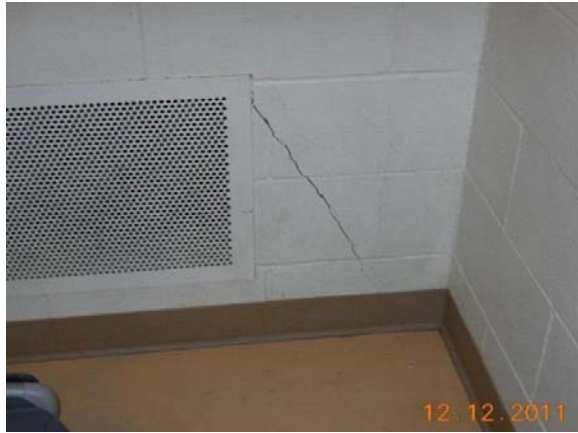
Figure 24A. Crack adjacent to vent in northwest corner of Gymnasium, Room F125. WSP Wall Movement History Rpt. page 67 of 141, photo date 12/12/2011
