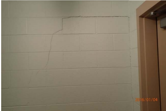
Figure 12A. Cracking in north bearing wall near joint with non-bearing wall in Room B171. M/M Presentation, slide 17, photo date 1/4/16
