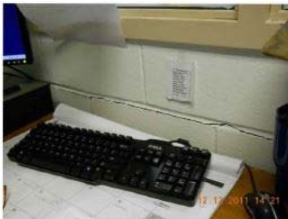
Figure 27A. Horizontal crack in masonry below window opening in Room F118. WSP Wall Movement History Rpt. March 31, 2015, page 3 of 141, photo date 12/12/11
