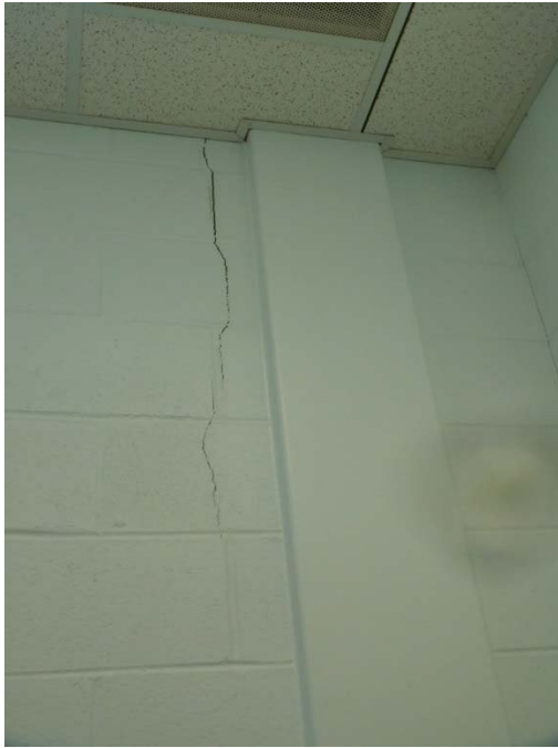
Figure 20. Vertical crack at intersection of non-bearing partition and column in Room D144
