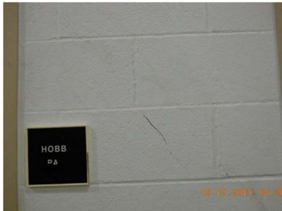
Figure 25A. Crack in CMU wall at entrance to Hobby/Craft Room F117. WSP Wall Movement History Rpt. page 67 of 141, photo date 12/12/2011
