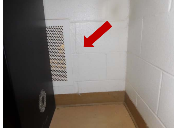
Figure 24B. Repaired (caulked) crack adjacent to vent in northwest corner of Gymnasium, Room F125. WJE Photo DSCN1446, date 6/22/2017
