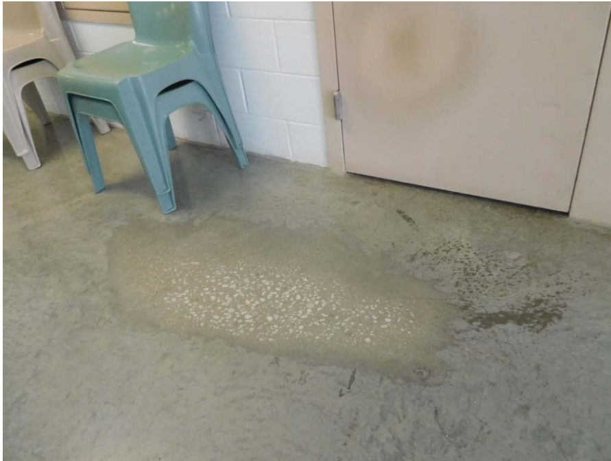
Figure 6. Indication of past grinding of slab surface to facilitate door operation
