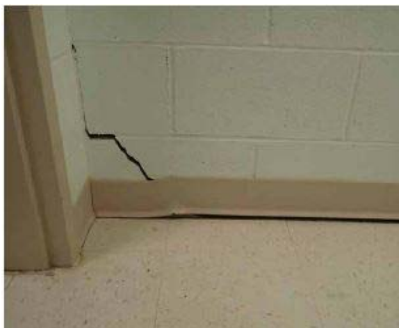
Figure 17A. Cracking in west non-bearing wall at juncture with bearing wall in Room B167. M/M Rpt. page 36 of 284, photo date 1/27/15
