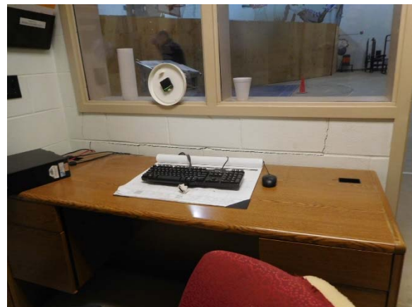
Figure 27B. Horizontal crack in masonry below window opening in Room F118.
