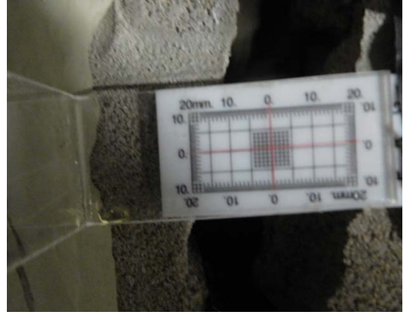
Figure 4B. Crack gauge 3 - Area F Near NE corner of Electrical Room F116.
