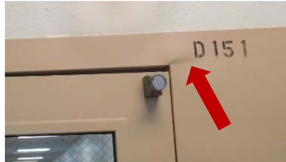
Figure 22B. Buckled metal door frame D151 in Corridor D151.
