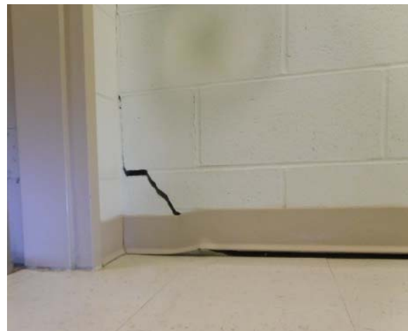
Figure 17B. Cracking in west non-bearing wall at juncture with bearing wall in Room B167. WJE Photo DSCN1226, date 6/15/17
