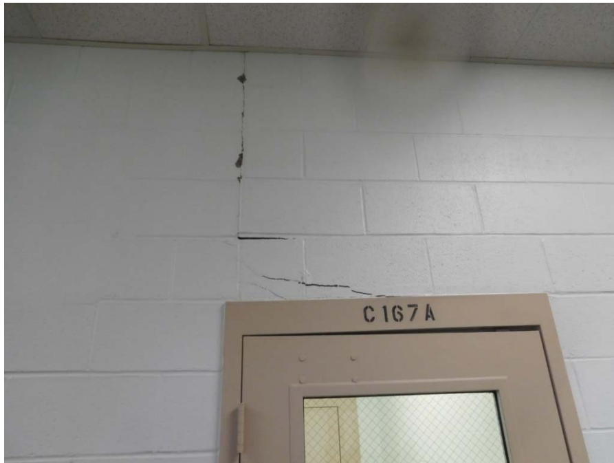
Figure 16. Racked door and distressed masonry
