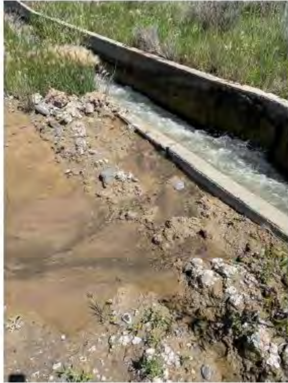
Figure 1. Observed water leaking through the chute wall
