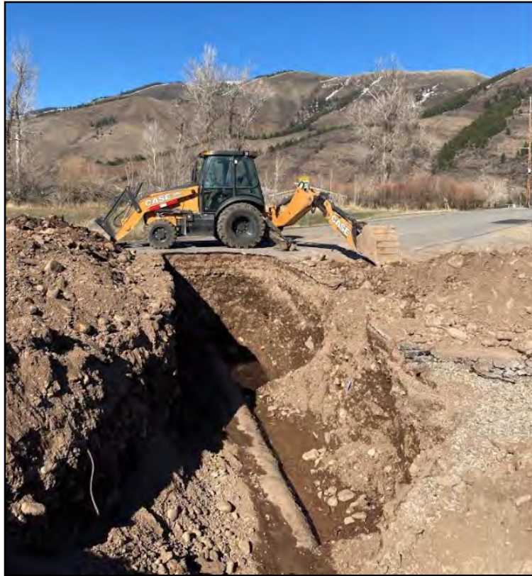
Pipe Conditions (top photos) and extent of ground disturbance typically required to repair leaks (bottom photo)
