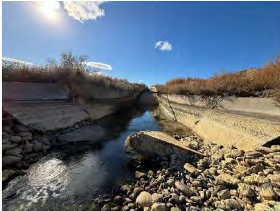
Figure 2. Movement in the drop structure walls
