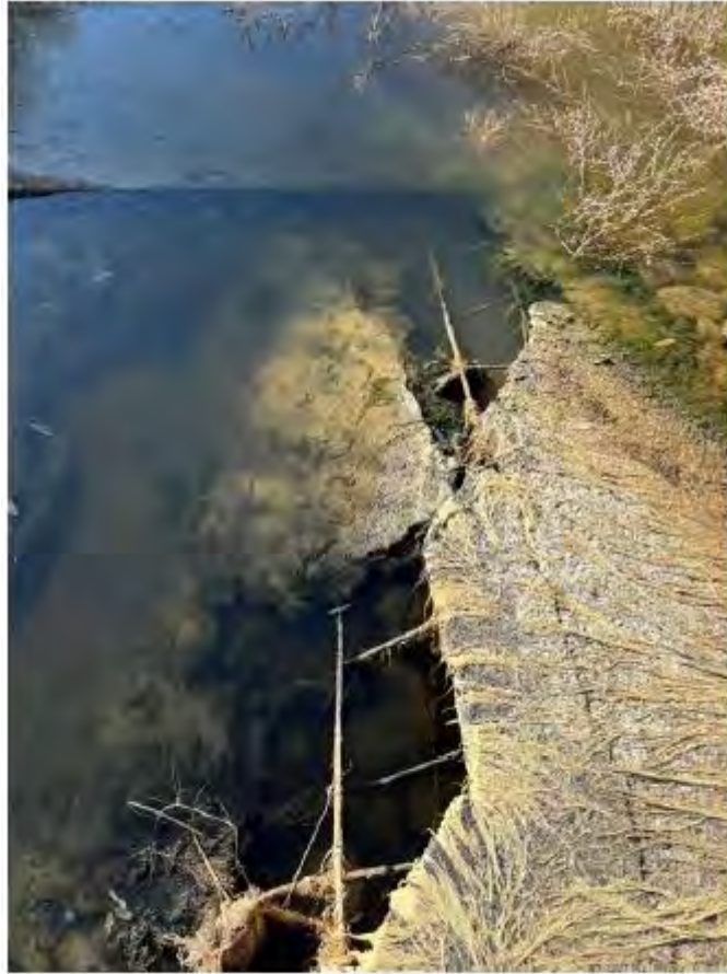
Figure 3. Large portions of the drop structure have broken
